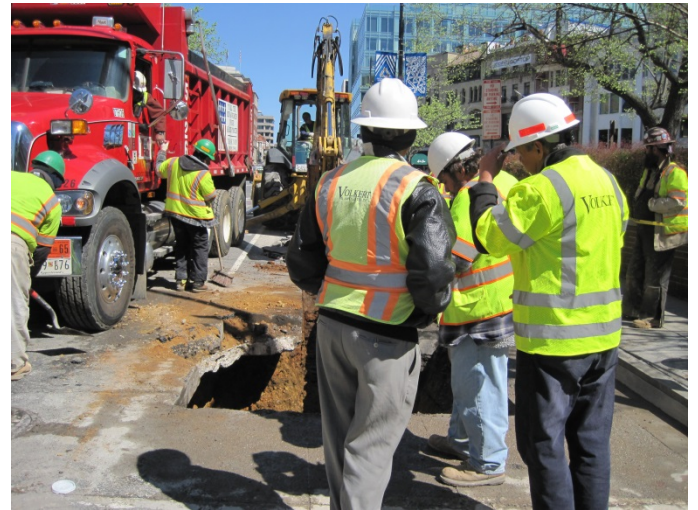
Volkert Inspectors at excavation site on the northwest side in the roadway at 18 th Street and M Street
