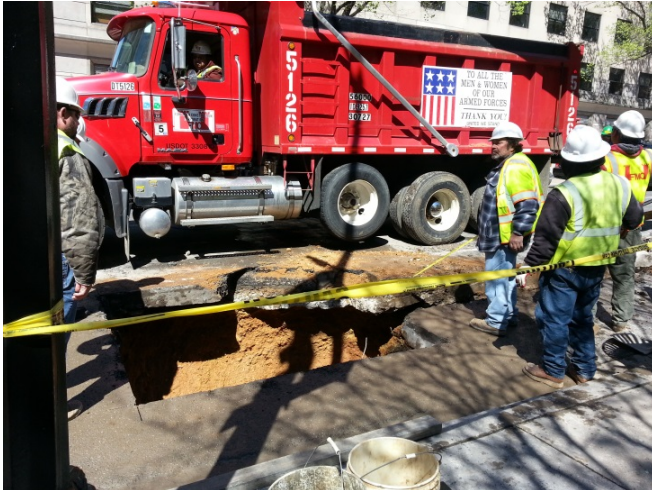
Excavation for a 4x4 manhole on the northwest side of 18 th Street between M and N Street
