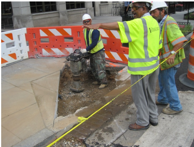
Volkert Inspector at sidewalk ADA ramp site on N Street and Connecticut Avenue
