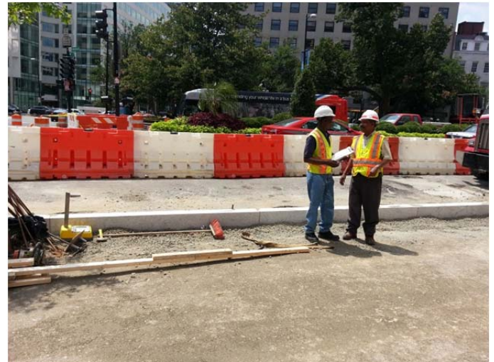
Volkert Project Engineer and DDOT Soils Lab Technician on Connecticut Avenue going northbound between M Street and N Street on the east side
