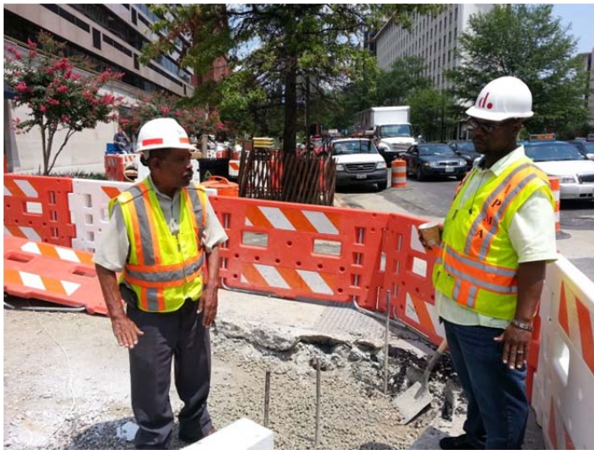
Volkert Project Engineer and DDOT Representative at sidewalk installation site on Connecticut Avenue going northbound between Rhode Island and N Street
