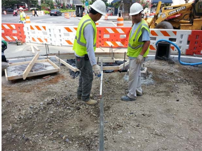
ADA Wheelchair ramp installation on the corner of M Street and Rhode Island Avenue on Connecticut Avenue on the east side
