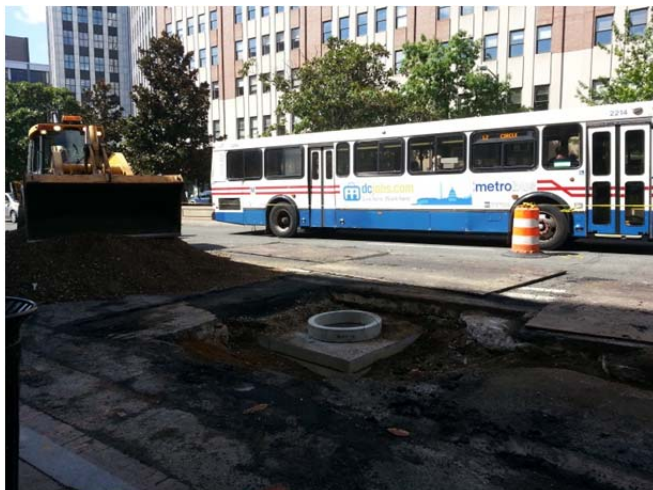
Manhole at the end of the trench excavation on the right lane on Connecticut Avenue between N Street and DuPont Circle
