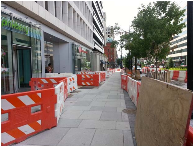
Completed pavers and pedestrian barriers in front of the businesses on the east side of Connecticut Avenue from Rhode Island Avenue to N Street
