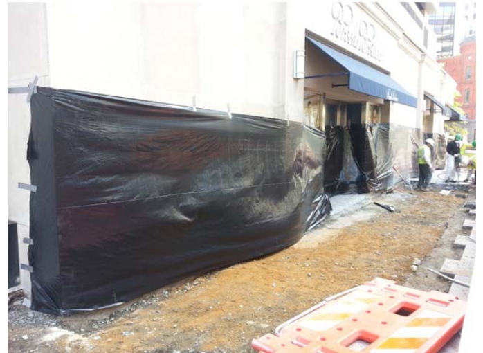
Protective covers before pouring concrete at the Brooks Brothers store at the corner of Rhode Island and Connecticut Avenue
