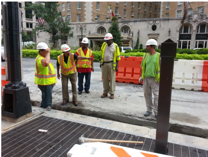
New FMCC Superintendent, Volkert Team, and DDOT Project Engineer at demo and curb/gutter installation on southbound Connecticut Avenue between L and M Street
