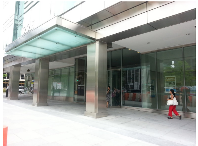
Completed paver installation on the east sidewalk of Connecticut Avenue in front of 1225 (World Bank Group)
