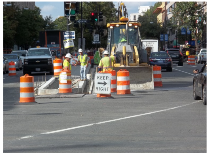
Median installation on Connecticut Avenue at the intersection of 18 th Street and N Street
