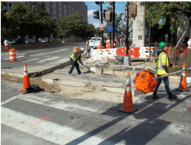
FMCC Flagger at wheelchair ramp, curb, and gutter installation on northbound Connecticut Avenue and N Street on the west side
