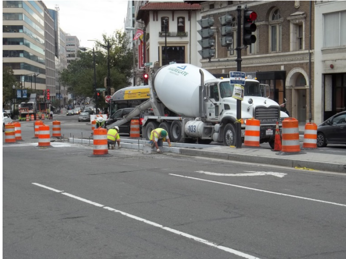
Median installation with new curb on Connecticut Avenue at the intersection of 18 th Street and N Street
