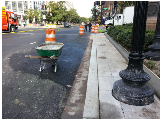
Curb and gutter installation on Connecticut Avenue and N Street at the John Witherspoon Park
