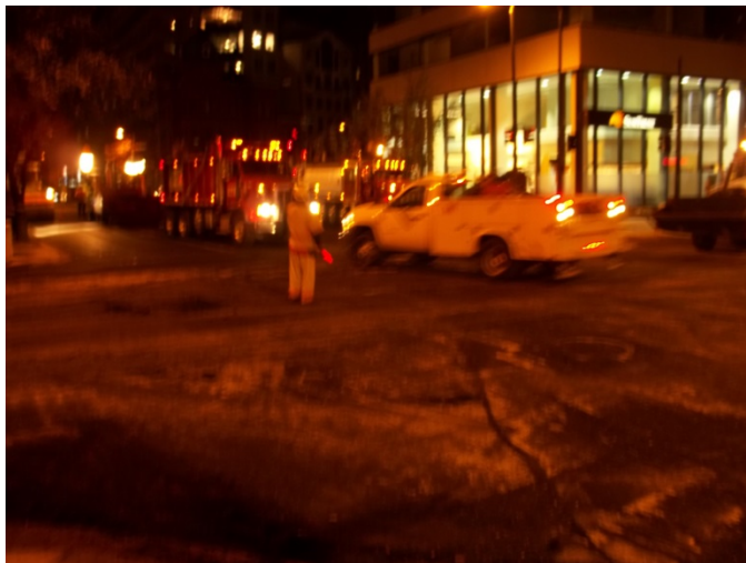
Night time milling and paving asphalt at the intersection of southbound Connecticut Avenue and M Street
