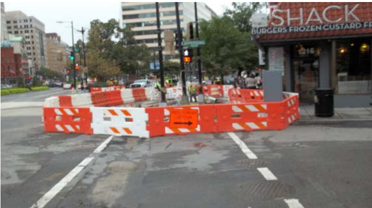
Working on sidewalk at the intersection of 18th St. and Jefferson Place after resolving a conflict with fire hydrant grade.
