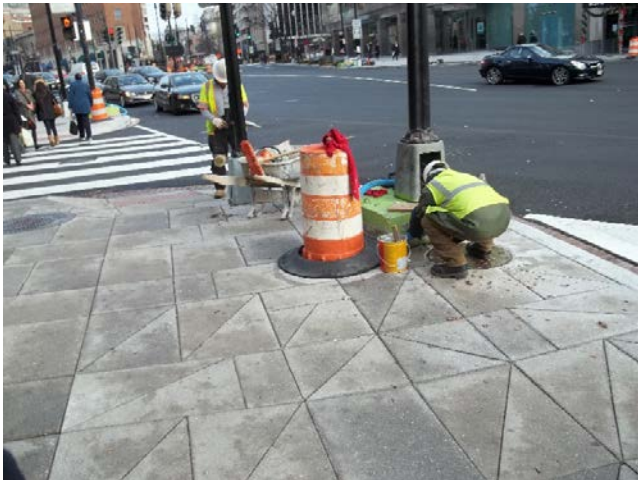
Applying water proofing sealant along the sidewalk near the southwest portion of the intersection at Connecticut Avenue and M Street.
