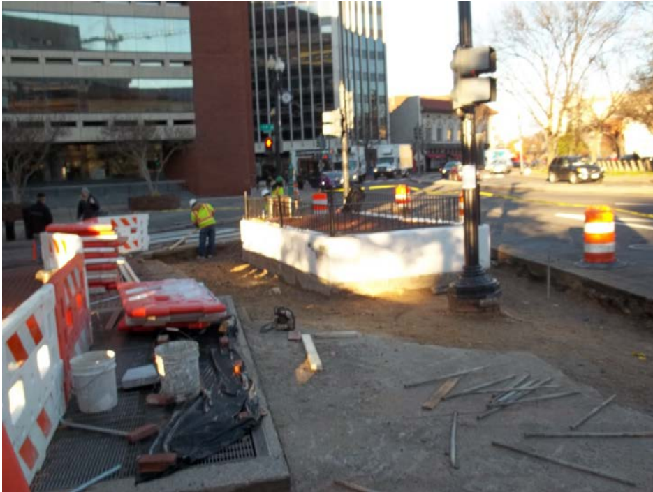
Demolition and construction lay out, along the sidewalk of DuPont Circle, at the southwest intersection of 19 th Street and Connecticut Avenue.
