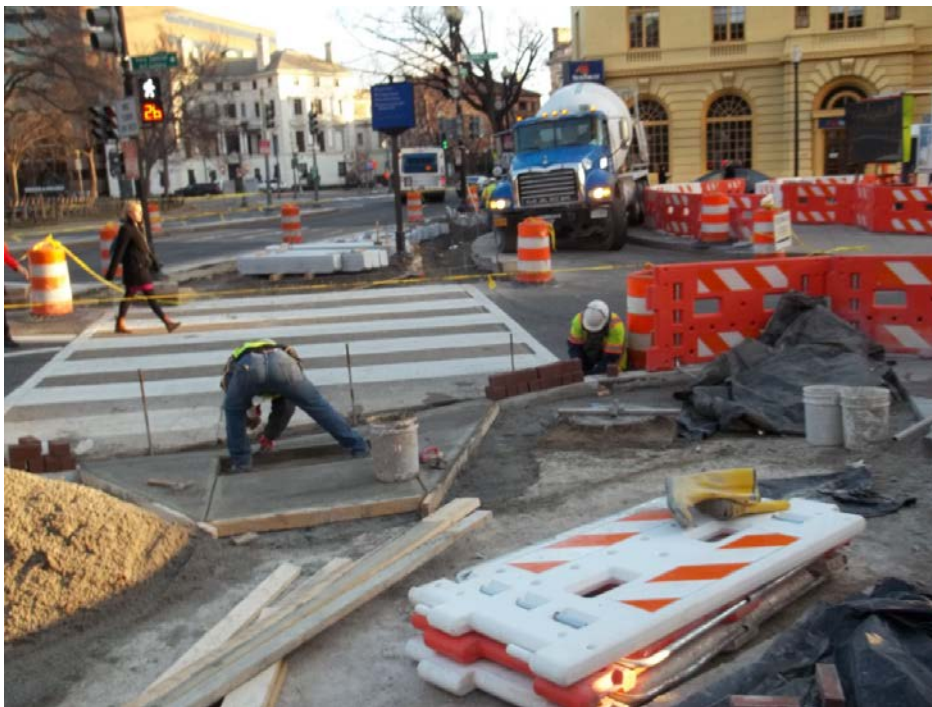
New handicapped ramp, located at the northeast corner, of the intersection between DuPont Circle and the southbound lanes of Connecticut Avenue.
