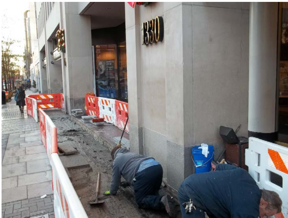
Applying water proofing treatment, under the sidewalk, in front of the entrance to Building #1330 on the southbound side of Connecticut Avenue.
