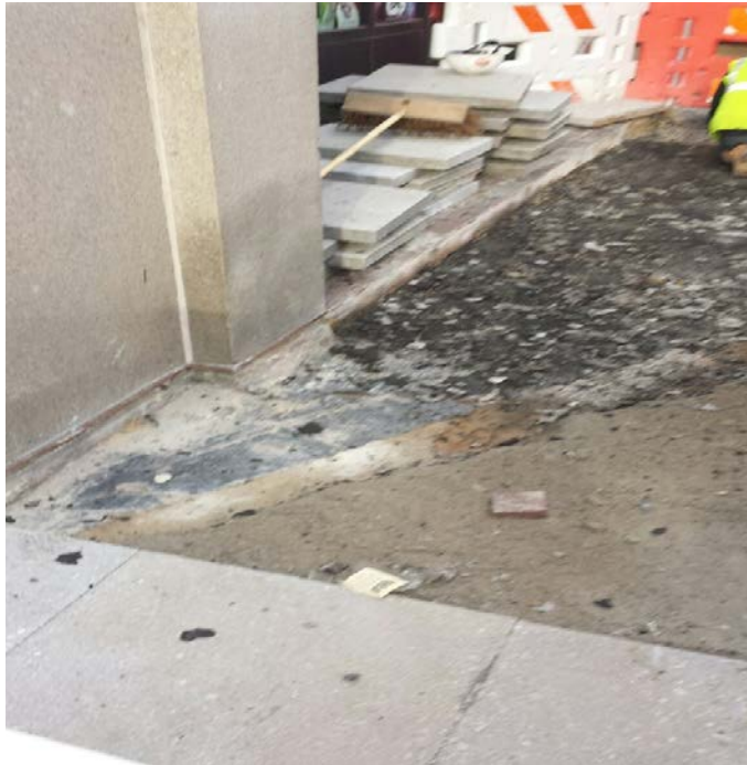
Brick paver removal and cleaning of concrete surface prior to the application of water proofing sealant along the entrance area of building #1330, southbound side of Connecticut Avenue.
