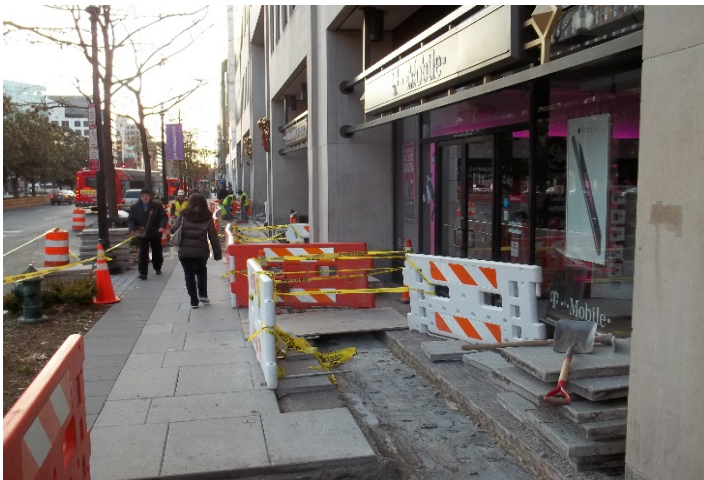
Water proofing operations, protected by plywood walk way planks and channelizers, at business entrances along Building #1330, southbound side of Connecticut Avenue.
