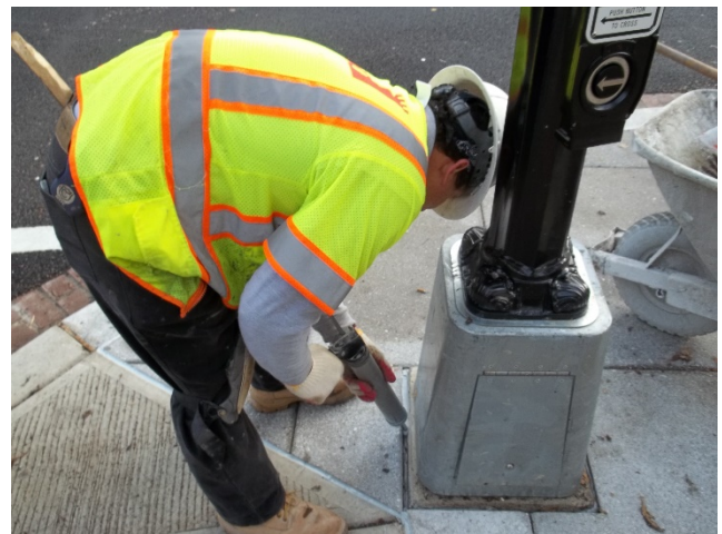
Water proofing sealant being applied around one of the bases of a light pole, located throughout the construction site of Connecticut Avenue.
