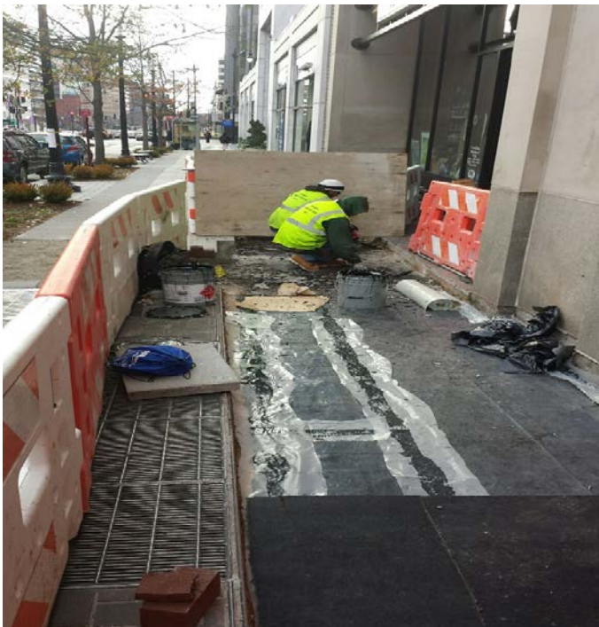
Cleaning of business entrance prior to the application of water proofing sealant, along one of the entrances, at building #1330, southbound side of Connecticut Avenue.
