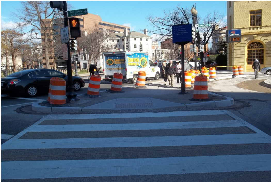
Completion of the curb, gutter, and handicapped ramps at the DuPont Circle and Connecticut Avenue parklet overlook.
