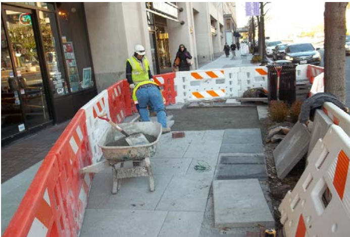
Replacement of sidewalk brick pavers, along the sidewalk in front of Building #1330, at the southbound side of Connecticut Avenue.
