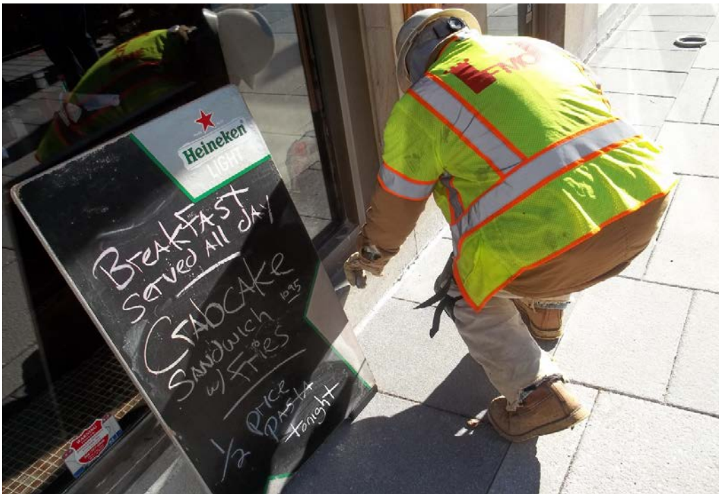
Placing expansion joint material and water proofing sealant, between the new brick pavers and existing buildings, along Connecticut Avenue.
