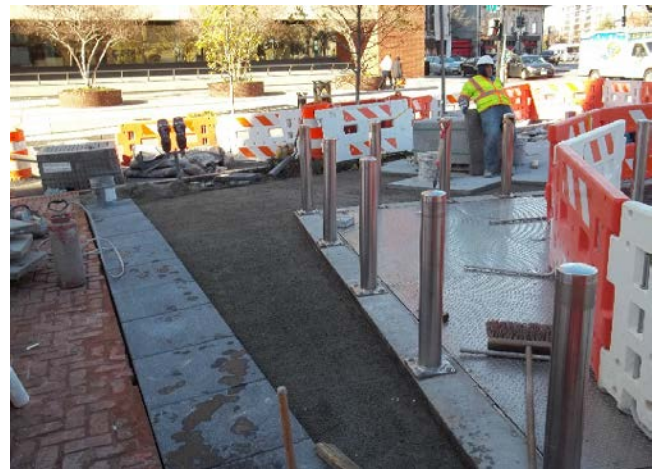
Placement of brick pavers, along the sidewalk, at the southern portion of the intersection of 19 th Street, Connecticut Avenue, and DuPont Circle.
