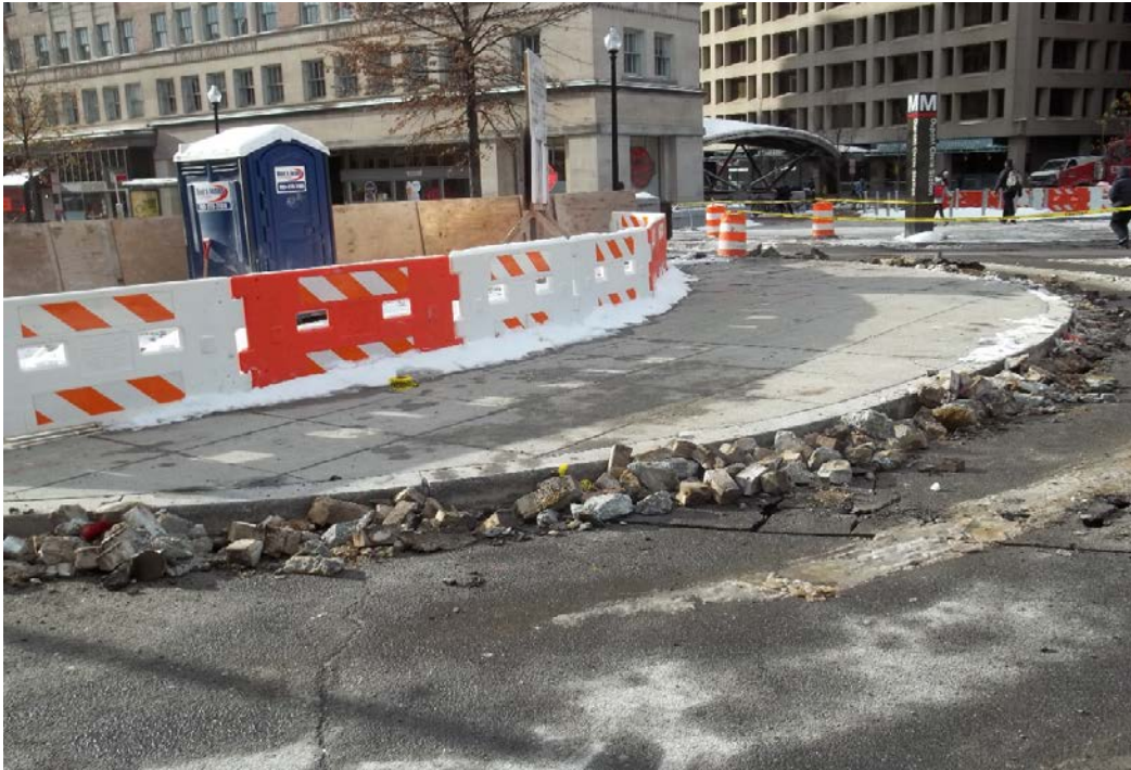
Demolition and excavation of the existing gutter along the turnaround of Connecticut Avenue at the southern portion of the intersection with DuPont Circle.
