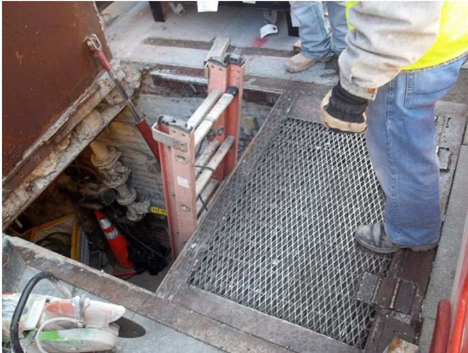
Removal of existing vault vent at existing vault gate at the 1300 Block of Connecticut Avenue.
