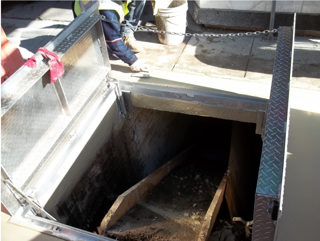
Adjustments to vault gate and assistance being provided to business owners with installation of existing cellar utilities.
