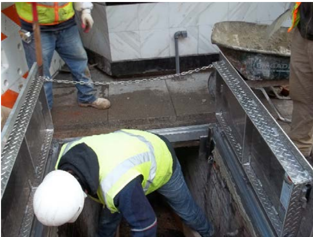
Inspection and cleaning of new vault gates along 1300 Block of Connecticut Avenue.
