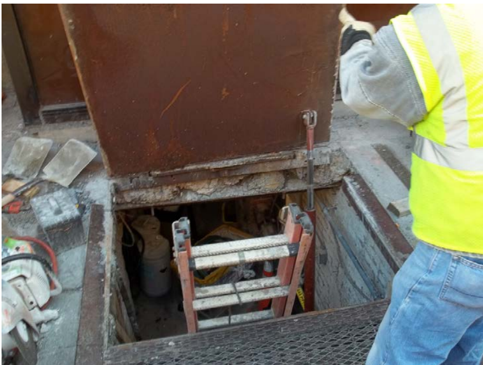
Preparation for removal and installation of a new vault gate along the 1300 Block of Connecticut Avenue.
