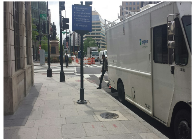
PEPCO service truck onsite to conduct service operations within the construction site.
