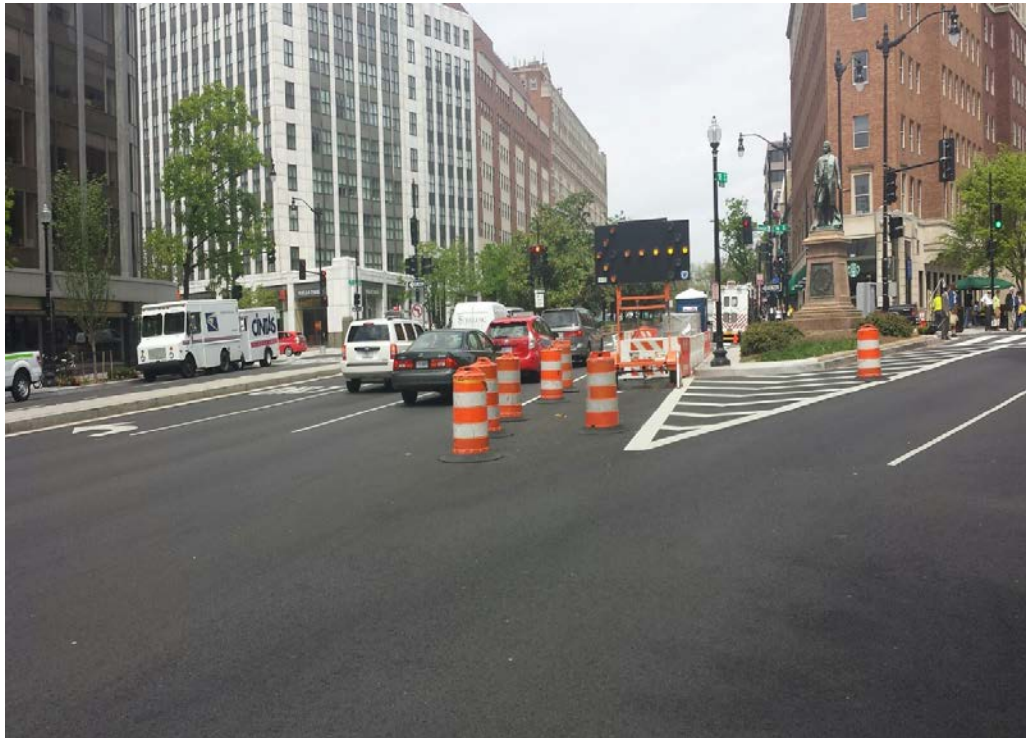
Work zone safety areas are delineated by using barrels and portable arrow boards, in order to direct traffic away from the construction zones.
