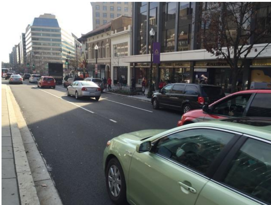
Volkert and contractor FMCC coordinate to address tightening bike racks and resolving tree fence repairs.
