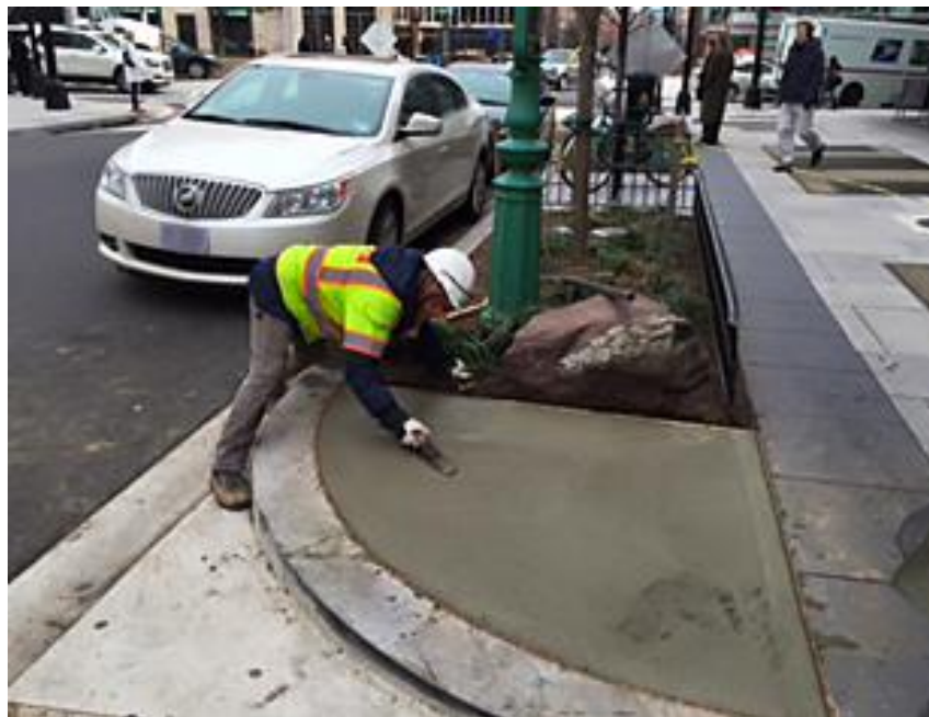
The additional concrete added adjacent to an entrance to address damage to the tree box area by vehicles.
